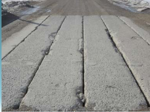
Gravel abrasion/worn edges on precast girders.
