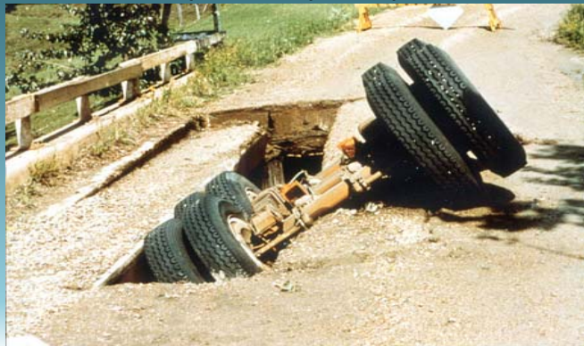
Consequence of pier cap failure.
