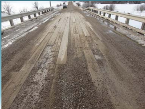
Worn/rotten timber strip deck.
