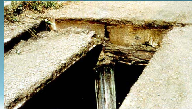
Collapsed girder where cap has failed.
