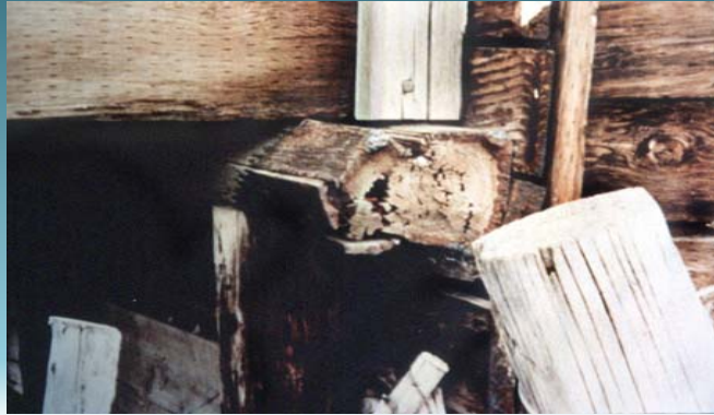
Rotten cap on abutment (bulging & crushing).
