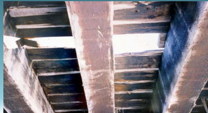
Rotten timber sub-deck.
