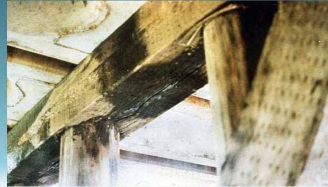
Pier cap crushing over piles.
