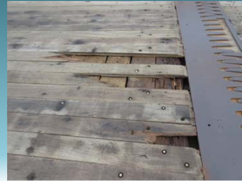
Missing and broken stripdeck
